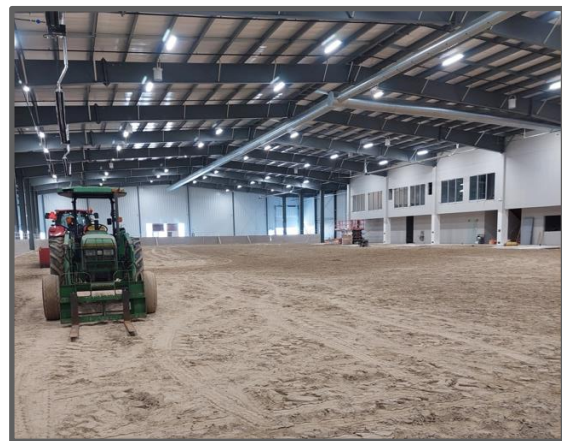
New equine facility under construction at Ancaster Fairgrounds, February 2022. Photo courtesy of Tina McNaughton
